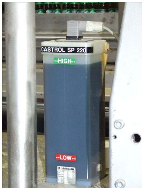
Figure 4: Visual Control for Packer machine's auto lube reservoir level
